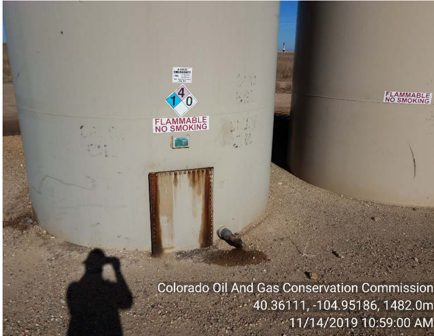
West crude oil tank leaks and stained soil on 11/14/19
