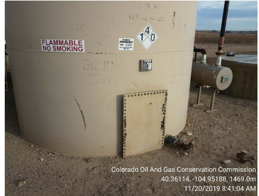
East crude oil tank leaks on 11/20/19
