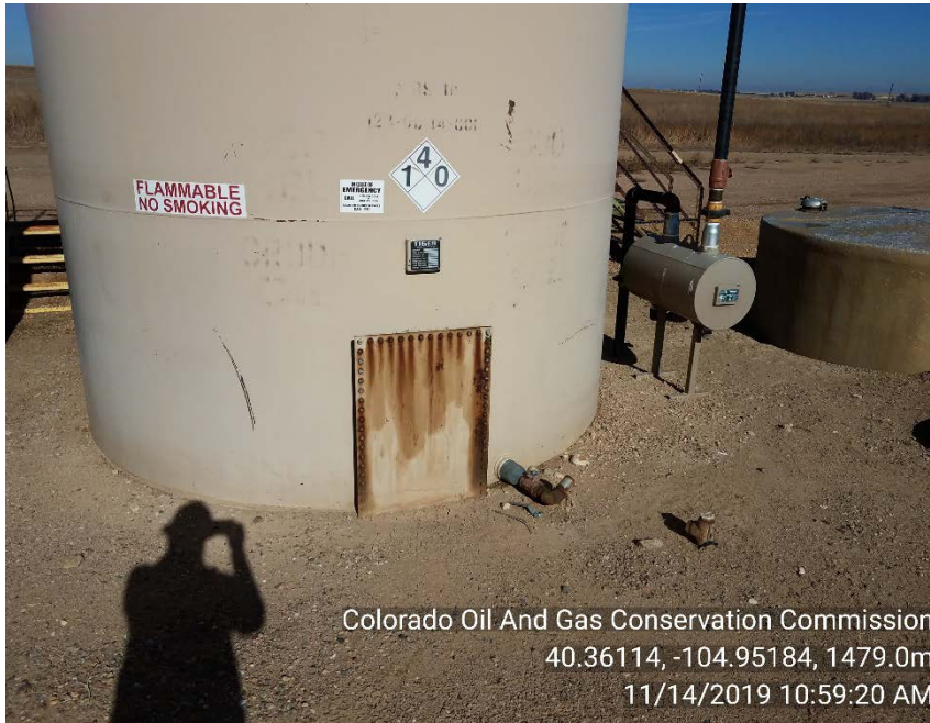
East crude oil tank leaks on 11/14/19
