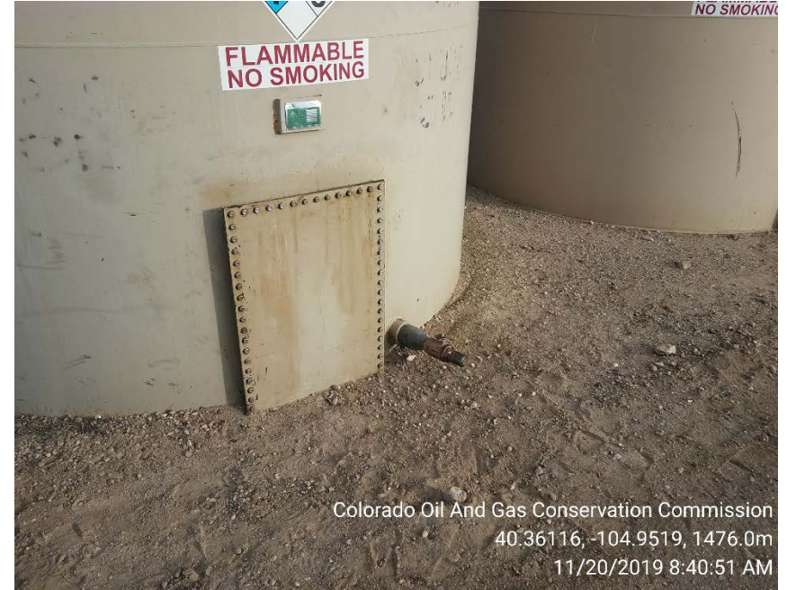
West crude oil tank leaks and stained soil on 11/20/19
