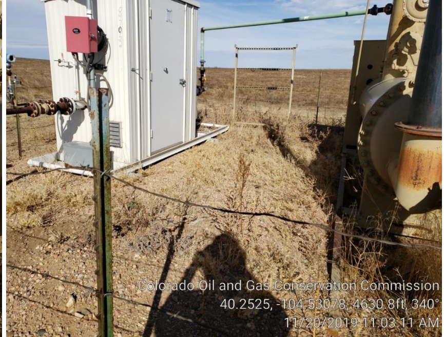
Photo #6 Weeds around Meter Run/ Separator. On 11/20/19
