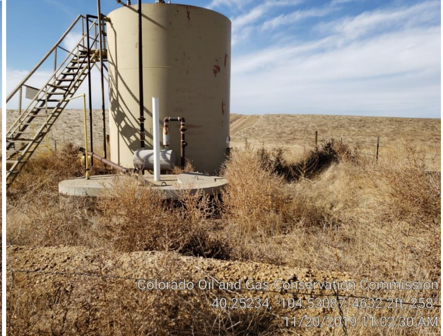
Photo #10 Weeds in Tank Battery. On 11/20/19
