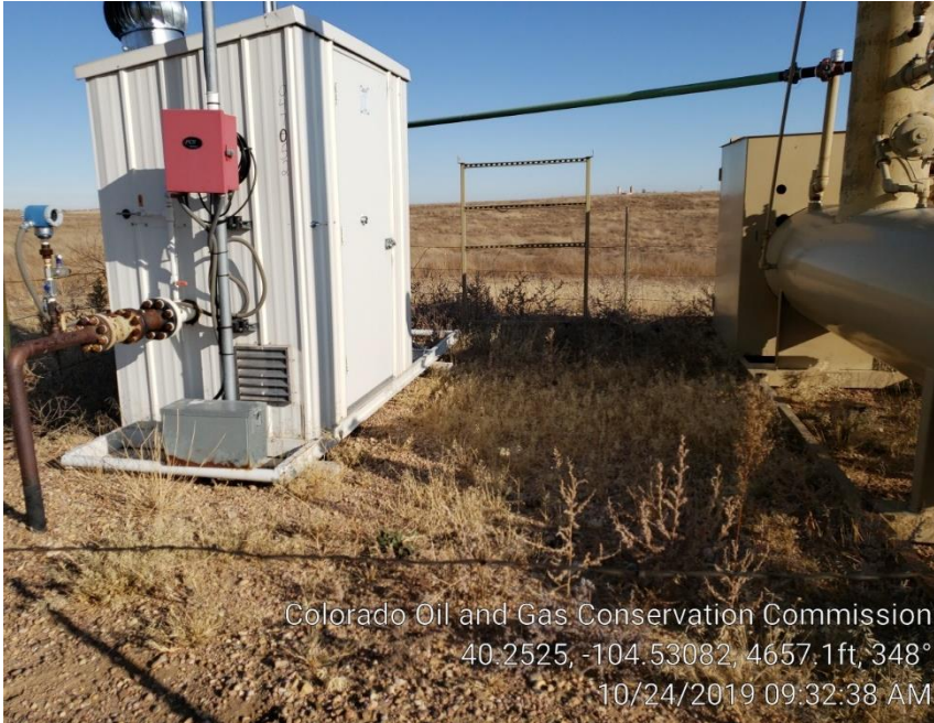
Photo #5 Weeds around Meter Run/ Separator. On 10/24/19
