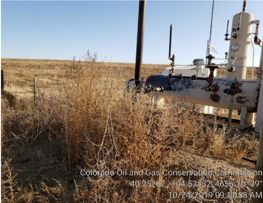
Photo #10 Weeds around Separator. On 10/24/19
