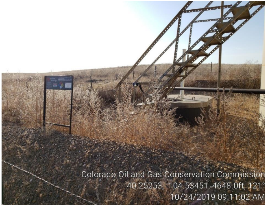
Photo #6 Weeds in tank battery. On 10/24/19
