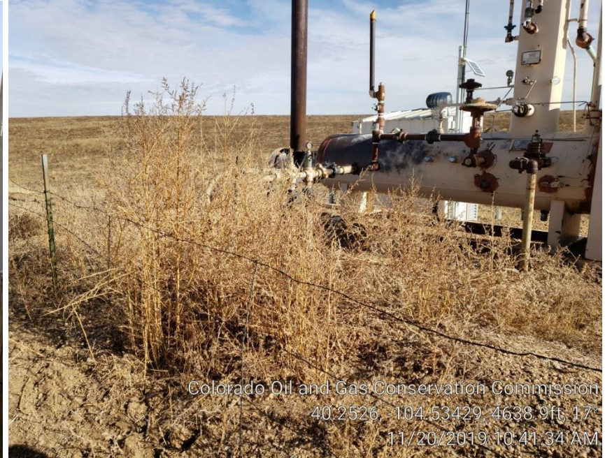
Photo #11 Weeds around Separator. On 11/20/19
