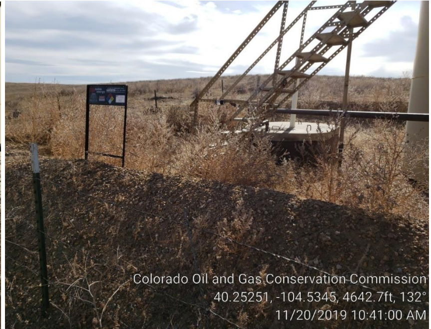
Photo #7 Weeds in tank battery. On 11/20/19
