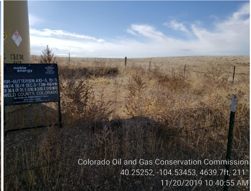
Photo #5 Weeds in tank battery. On 11/20/19
