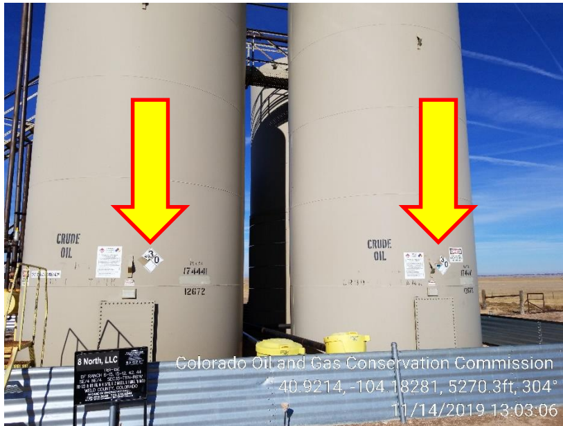
Photo 3 – South Tanks missing capacity and NFPA labels are peeling
