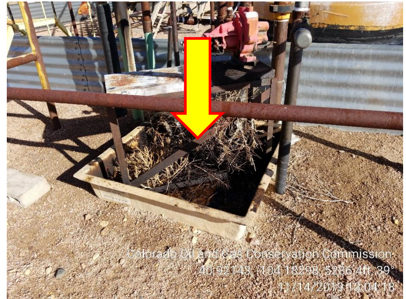
Photo 4 – Recycle Pump containment - Oily Waste and Wildlife protection devices not adequate
