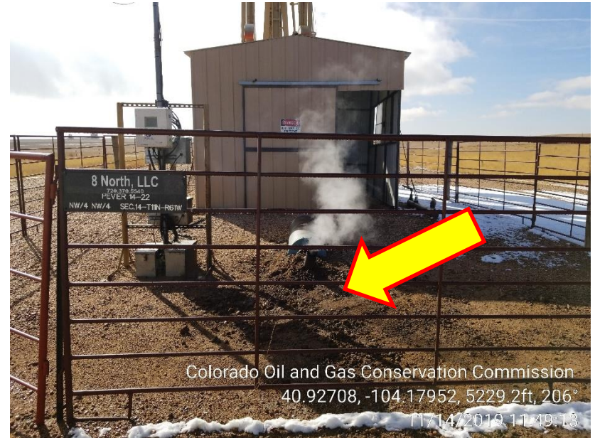
Photo 2 – Wellhead Sign. Stained Soil at Exhaust
