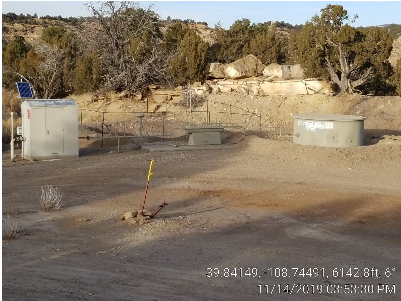
Photo 2. Separator, meter building, pit, and tank.
