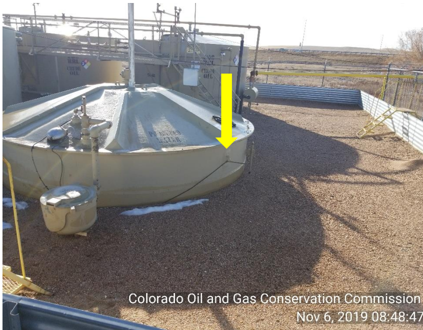
Photo 5 Flood plane anchors on produced water tank
