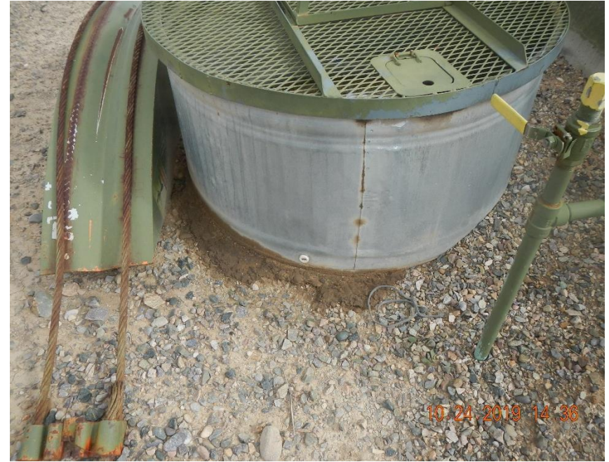
Stained soil at base of secondary containment for lube oil container.
