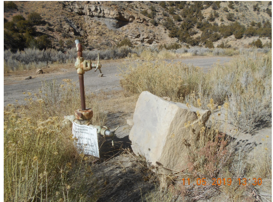
Temporarily Abandoned wellhead with sign.
