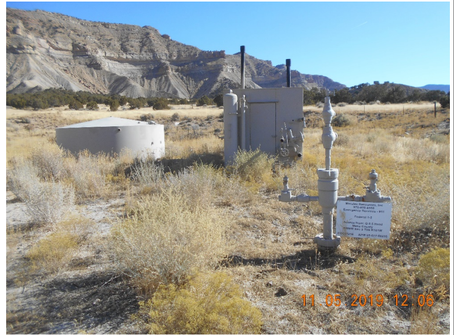
Temporarily Abandoned wellhead with sign, Separator and Tank disconnected.
