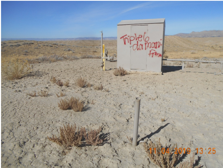
SW anchor and Meter housing with sales line riser. Looking N.
