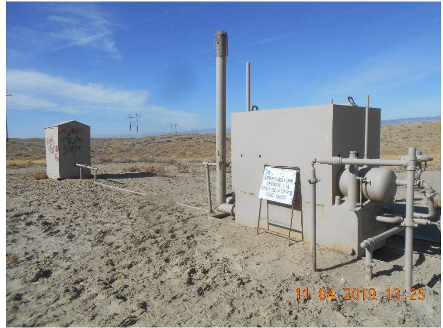
Separator and Meter housing with sign looking W
