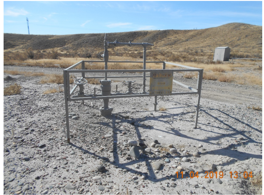
Wellhead with fence.
