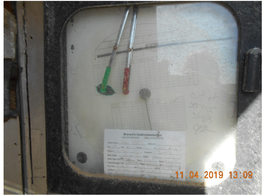
Meter with Out of Service label Dated 3/19/13
