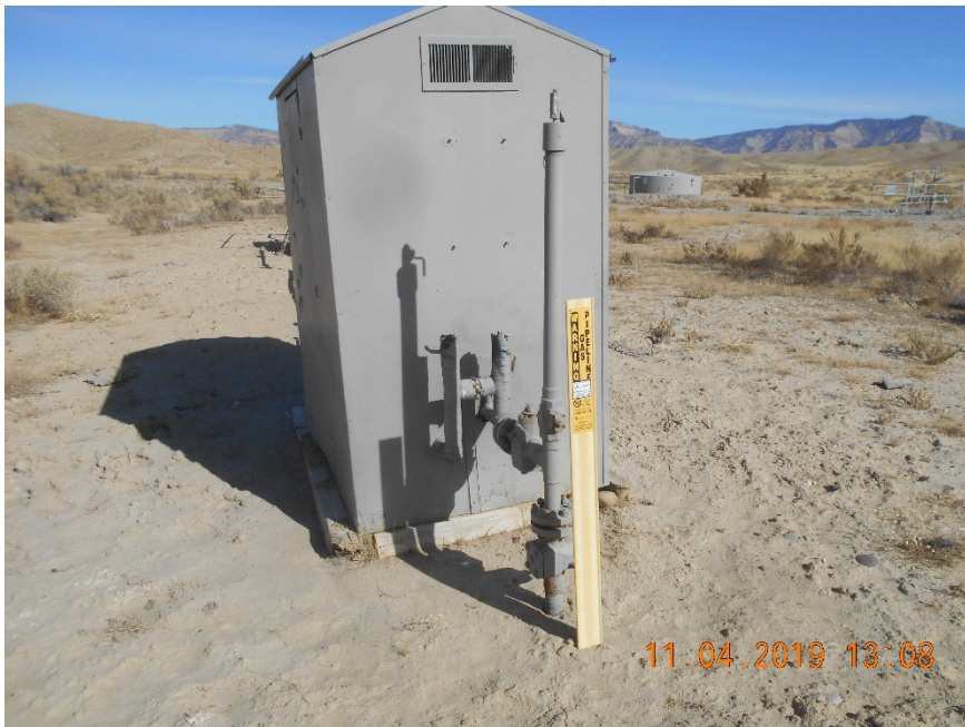
Meter housing with sales line riser.
