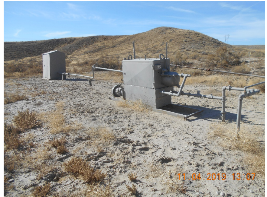
Separator and Meter housing looking SW
