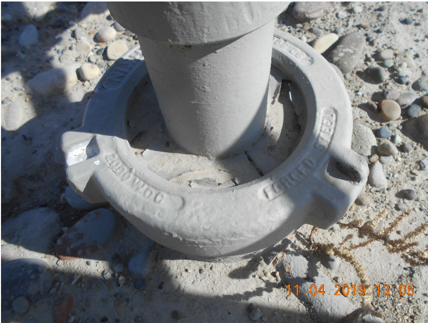
Audible leak at Surface casing / Production casing seal.
