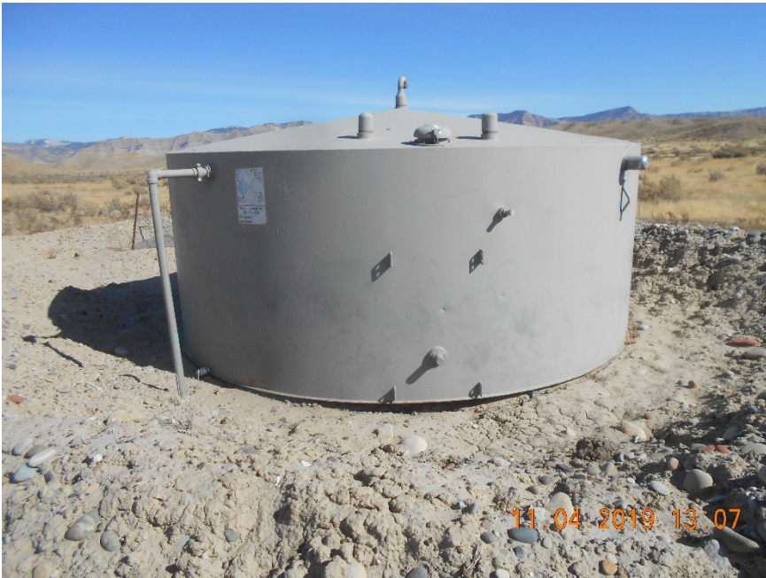
Produce water tank with fade and peeling labels.
