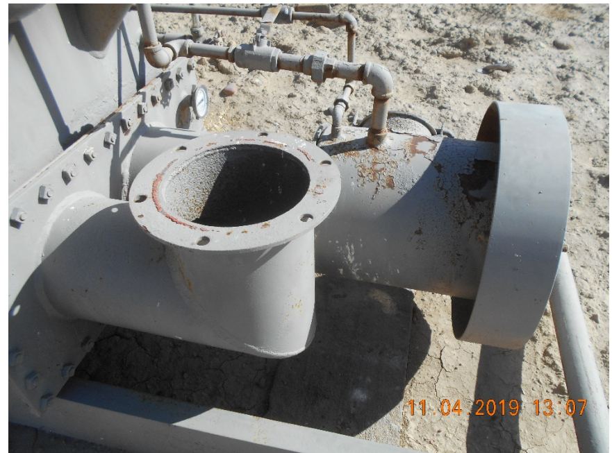
Open ended burner flue on separator with no bird/wildlife screen.
