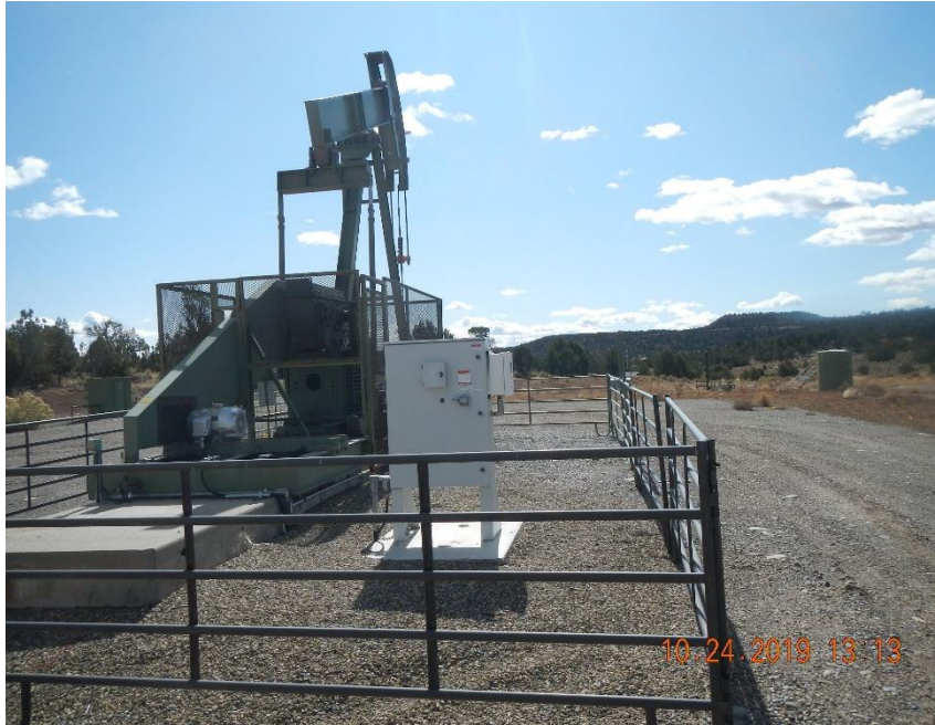
Electric prime mover.
