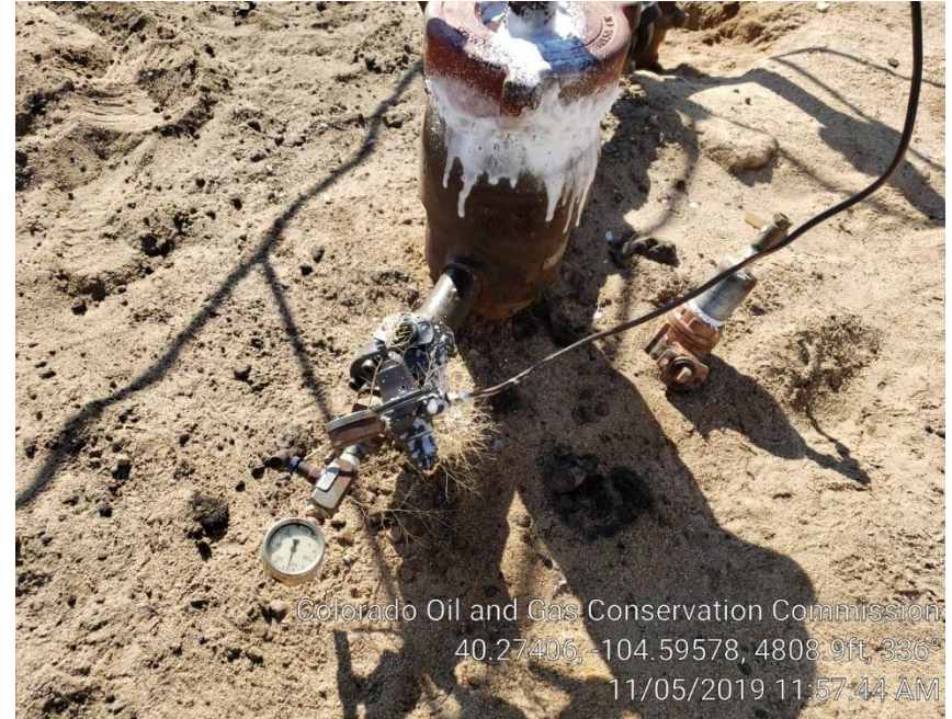
Photo #5 No Active leak at the Meco regulator stainless fitting. On 11/5/19
