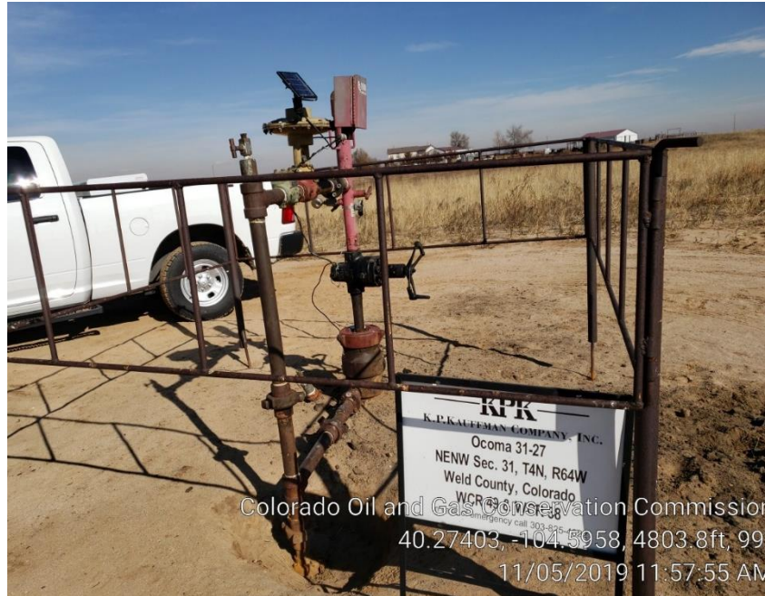
Photo #1 Wellhead & Sign
