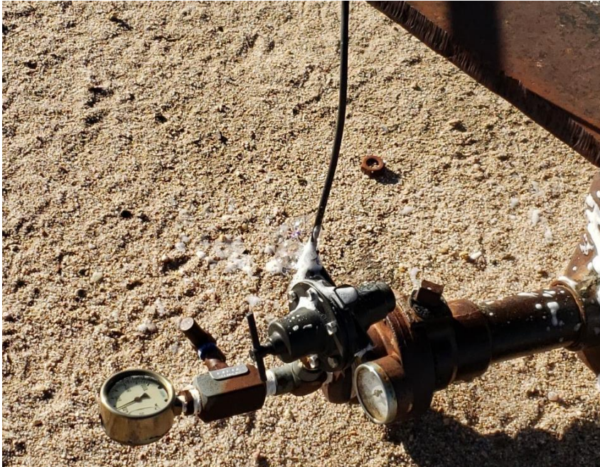
Photo #4 Active leak at the Meco regulator stainless fitting. On 9/26/19
