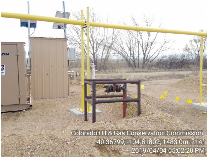
Photo #3 Mossberg-PM J30-9, Mossberg PMJ 30-10 Battery Unused Equipment Gas Meter run riser prior insp.
