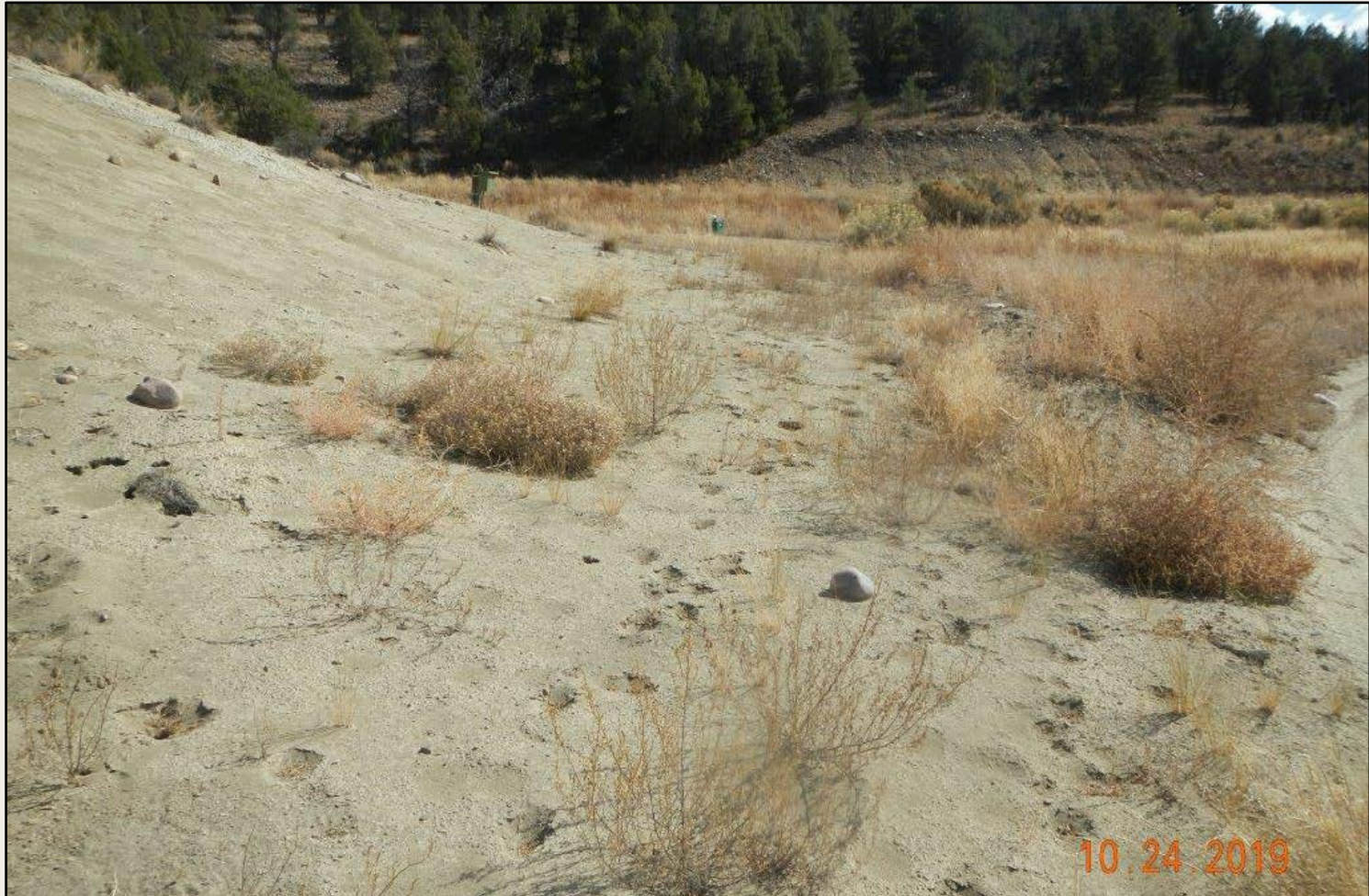
Photo 3. View of sediment deposition at the toe of the eastern cut-slope.
