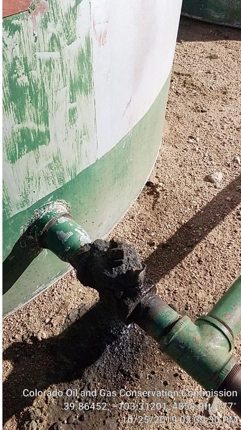
Mechanical conditions, north tank valve leak.
