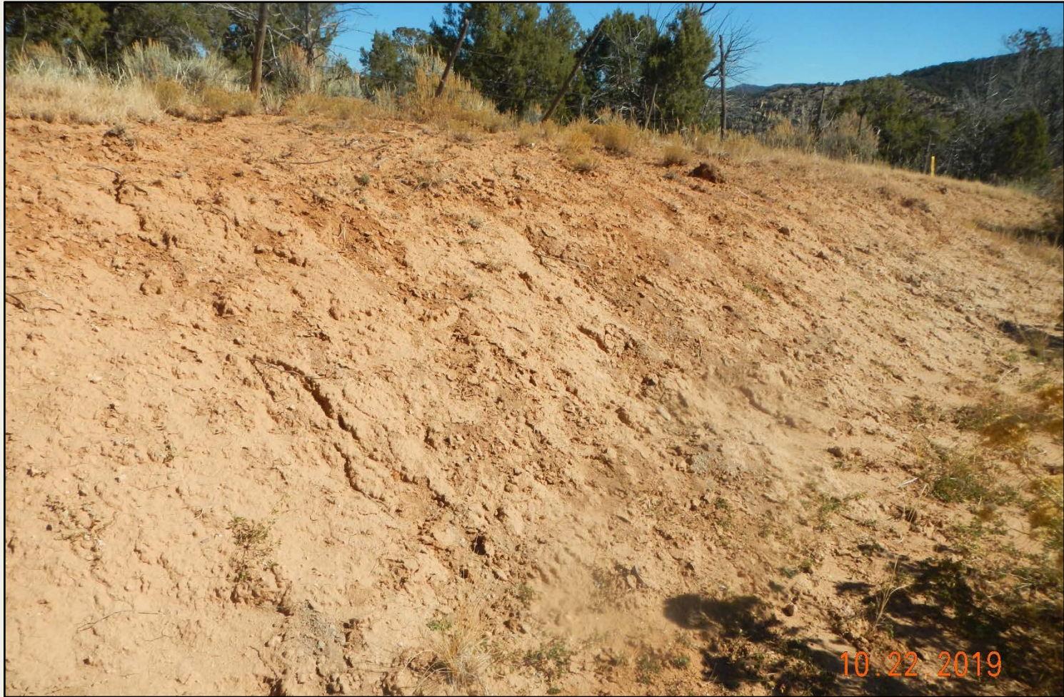
Photo 5. View of bare and eroding cut-slope within the northern project area.
