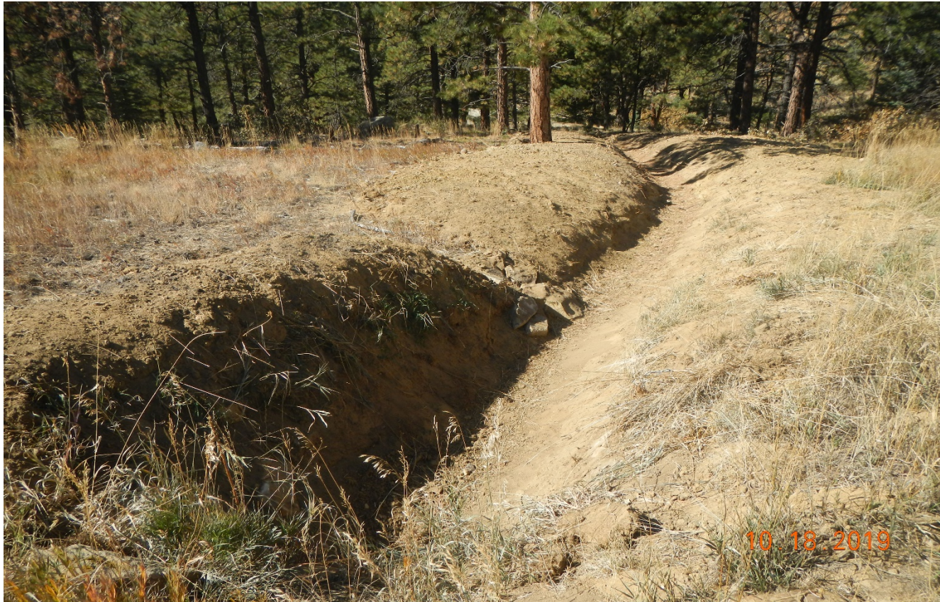
Photo 2. The culvert outlet and inlet were cleaned out of sediment buildup. Ditch has been excavated for stormwater drainage.
