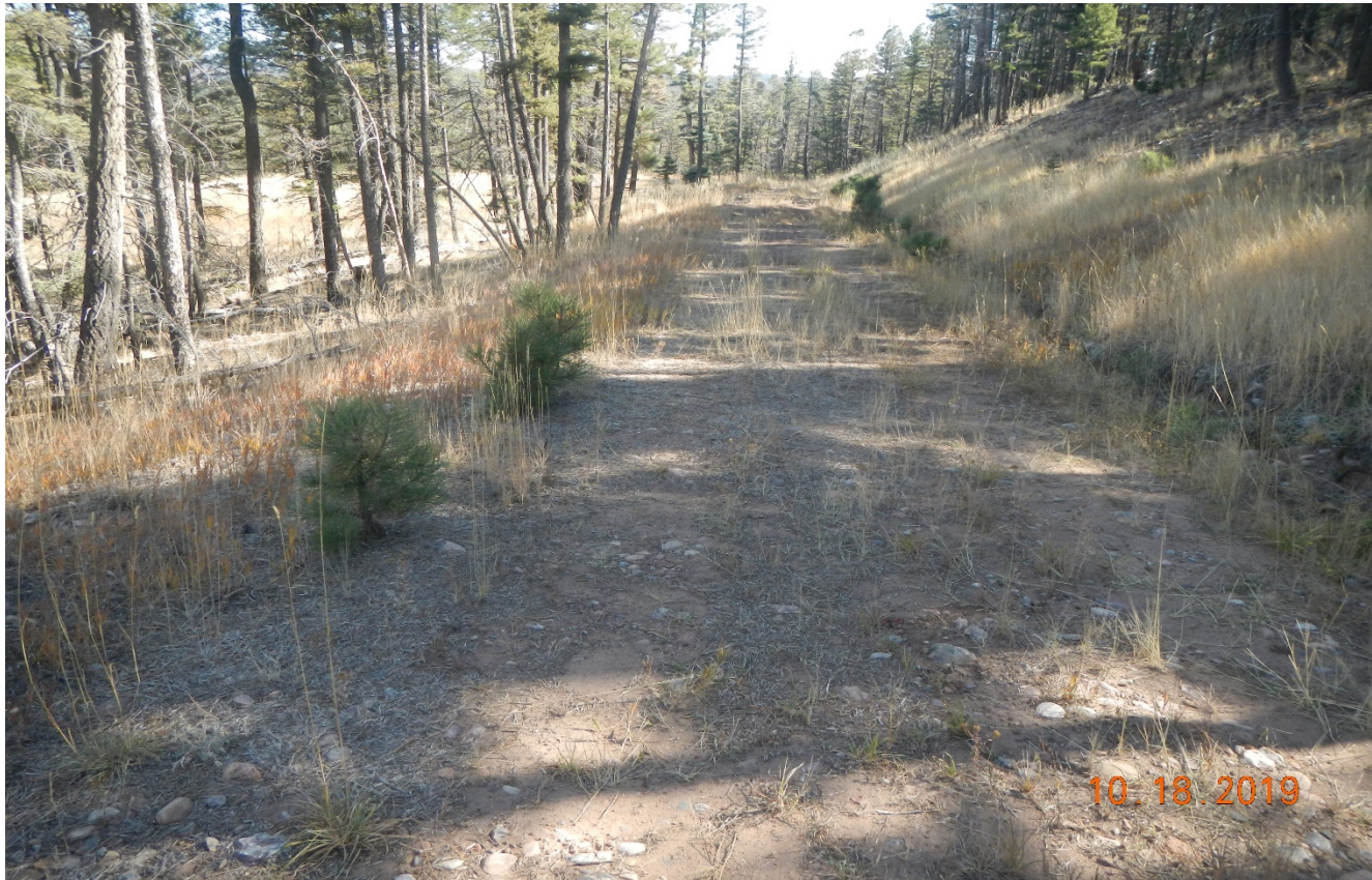
Photo 2. Facing northeast along the access road. Vegetation is well established along the road and culverts are maintained..
