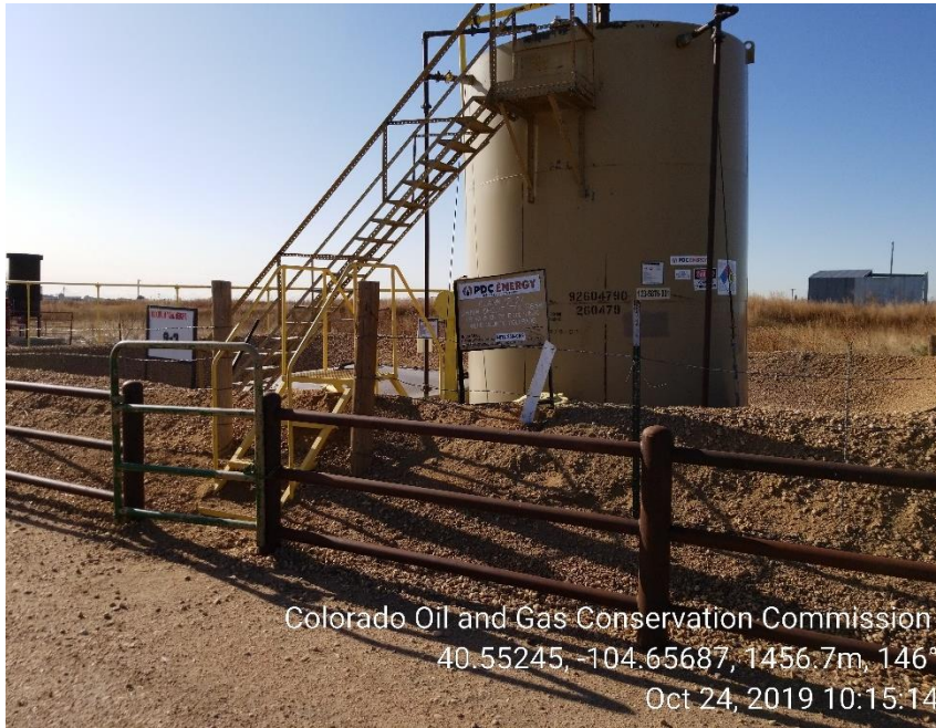
Photo 3: Centralized Tank Battery
