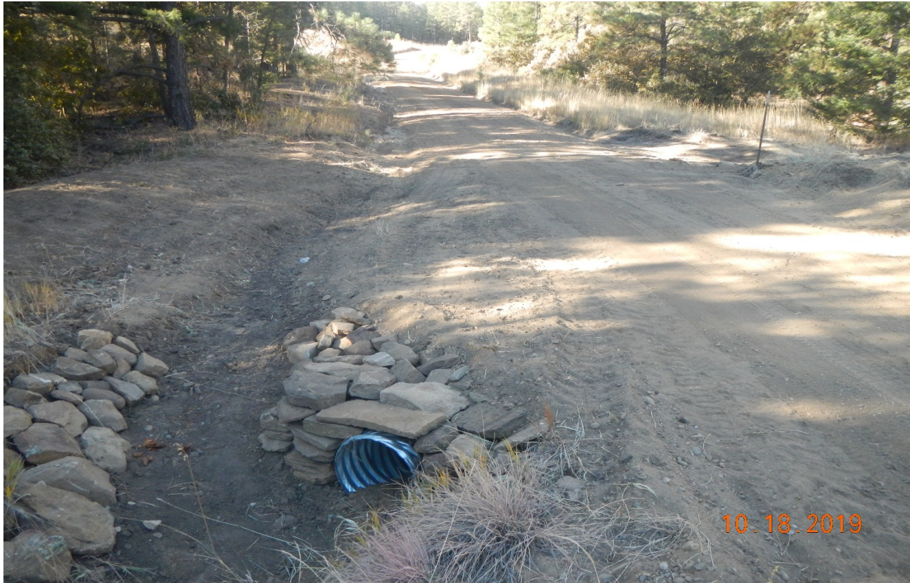
Photo 2. The culvert has been maintained along the road and the access road has been graded.
