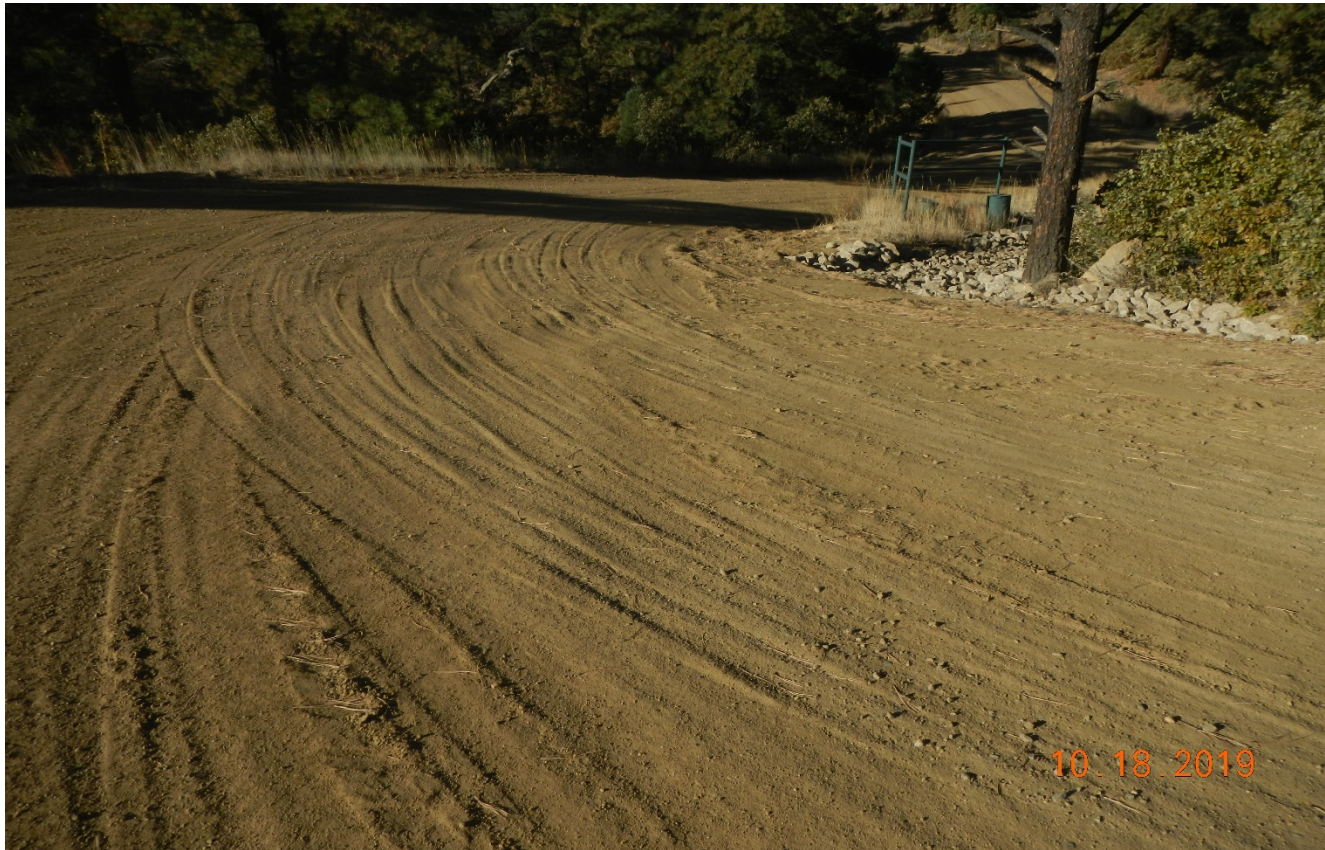
Photo 2. The erosion on the road near the location has been repaired. Rock rip/rap was installed along the side of the road. There is loose soils along the road from grading which may be susceptible to erosion.
