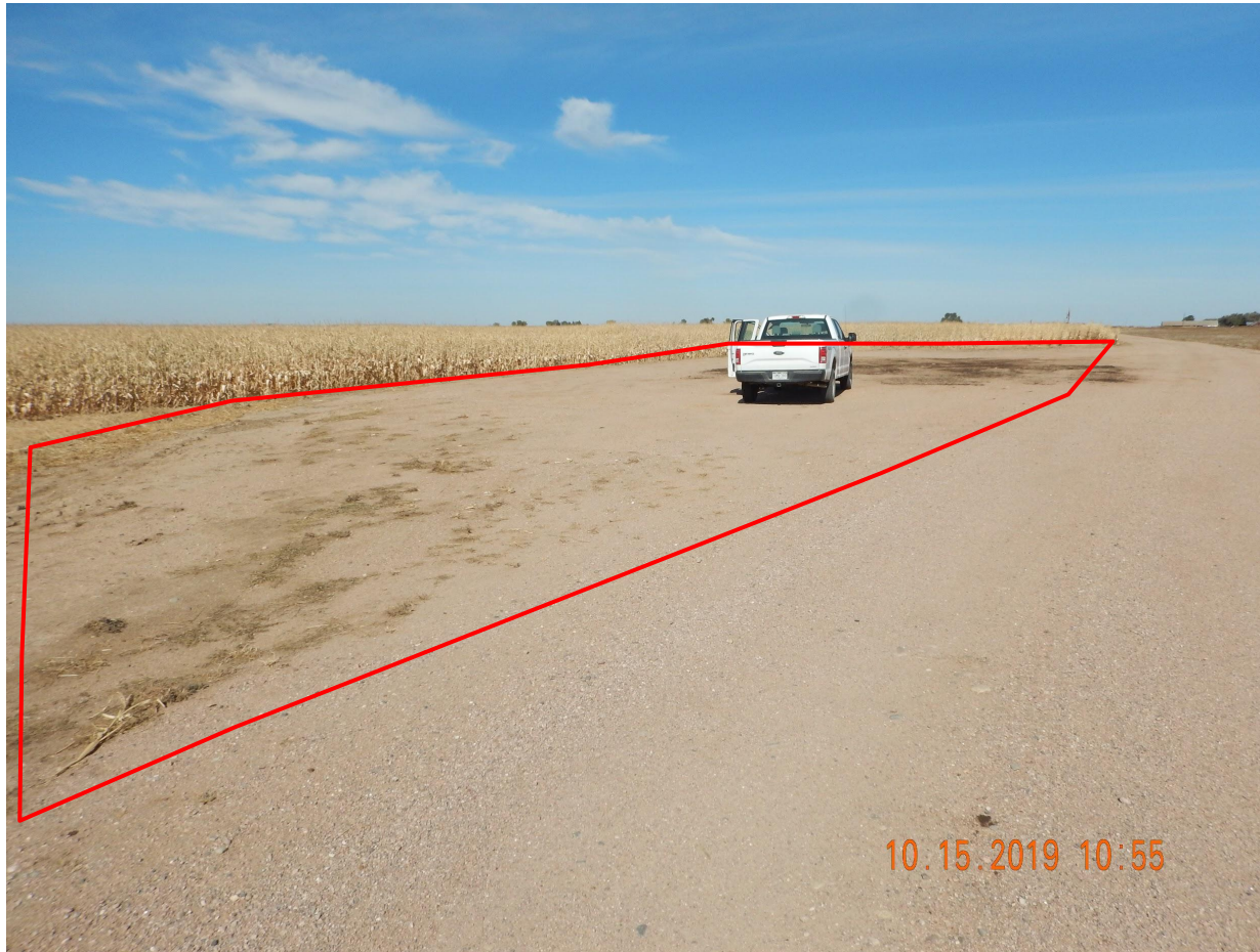
Photo 1. Photo taken from the southern location, facing North. Operator has failed to perform final reclamation activities at the location (i.e., remove gravel, decompact, seedbed prep and seed).
