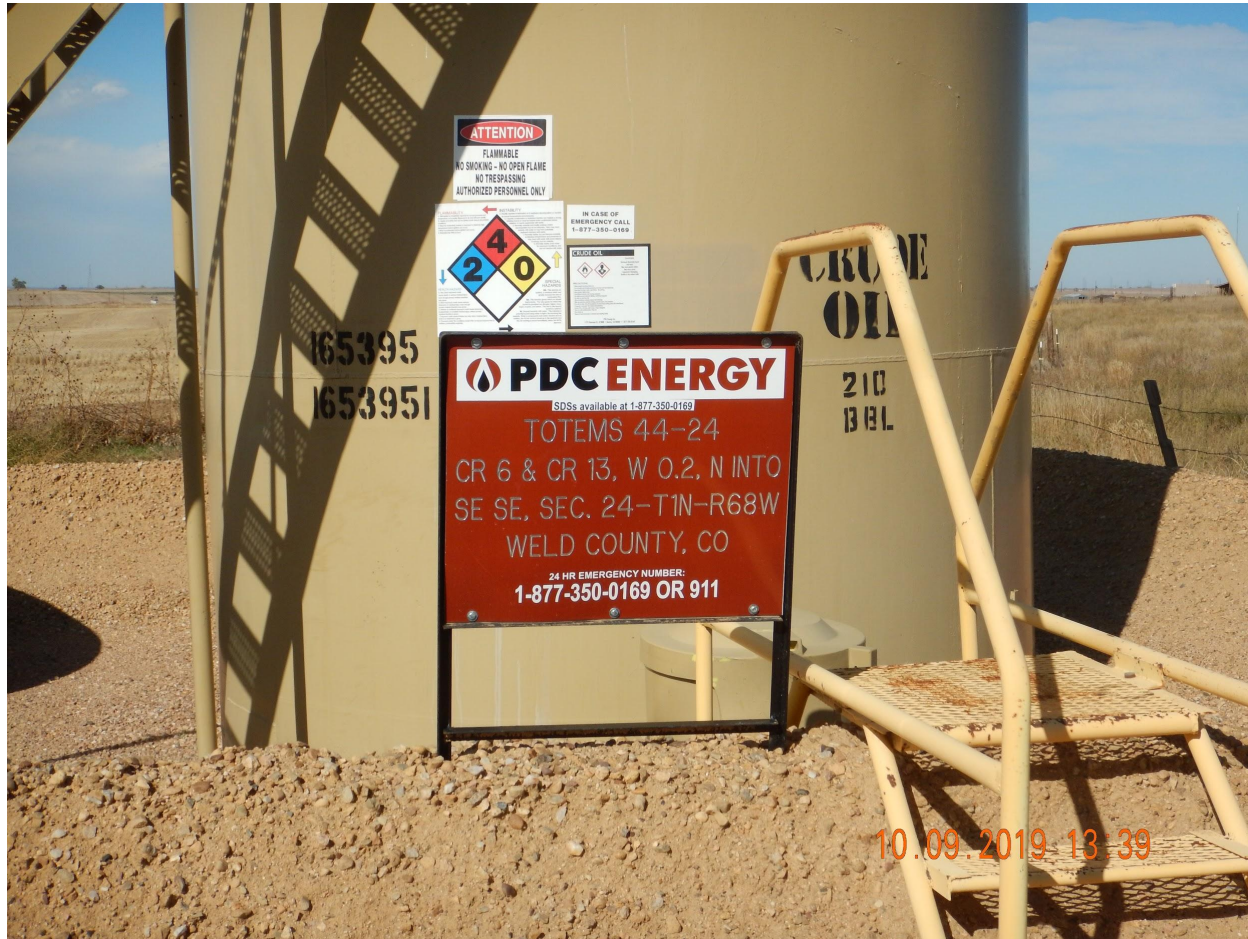
Photo 2. Photo taken from the associate tank battery location. Photo illustrates the tank battery is still in use for another nearby active well.
