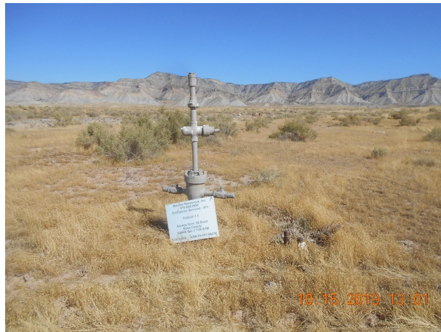
Wellhead with sign
