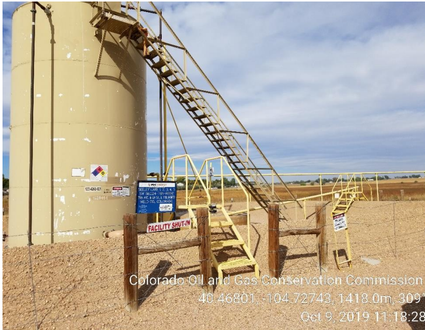
Photo 5: Centralized Tank Battery
