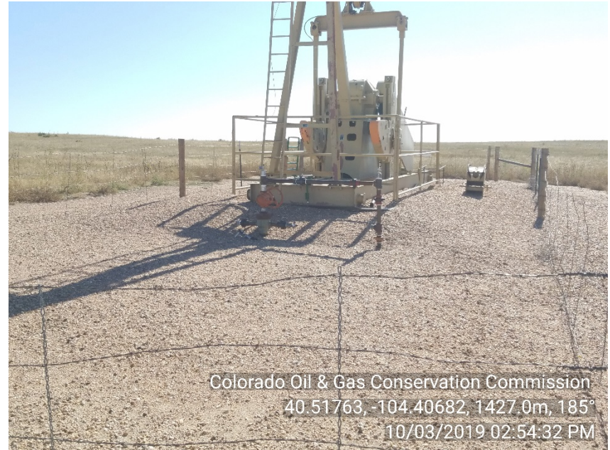
Photo #2 Brown 22-2 Wellsite Shut-In | SI
