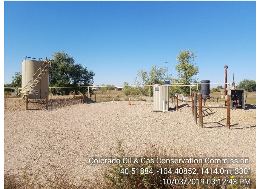
Photo #4 Brown 22-2 Battery Shut-down | Inactive
