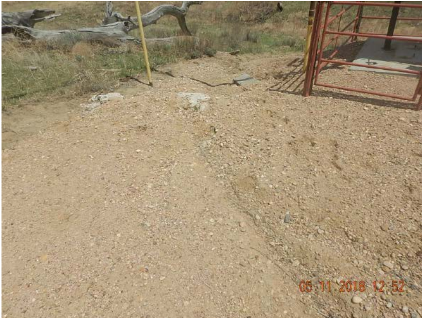
Photo #5 Brown 22-2 Battery NE Corner – Stormwater erosion prior insp.
