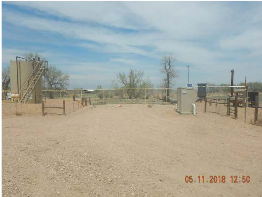
Photo #3 Brown 22-2 Battery Shut-down | Inactive prior insp.
