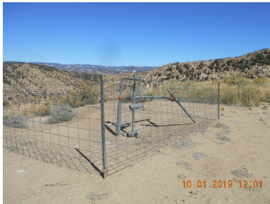
Wellhead with fencing.
