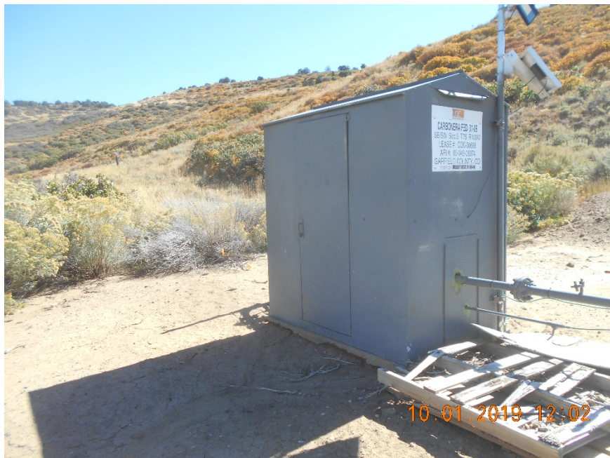
Meter Housing with sign
