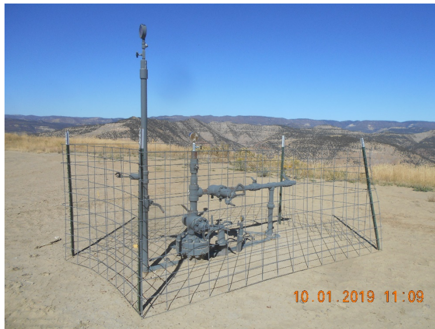
Wellhead with fencing.
