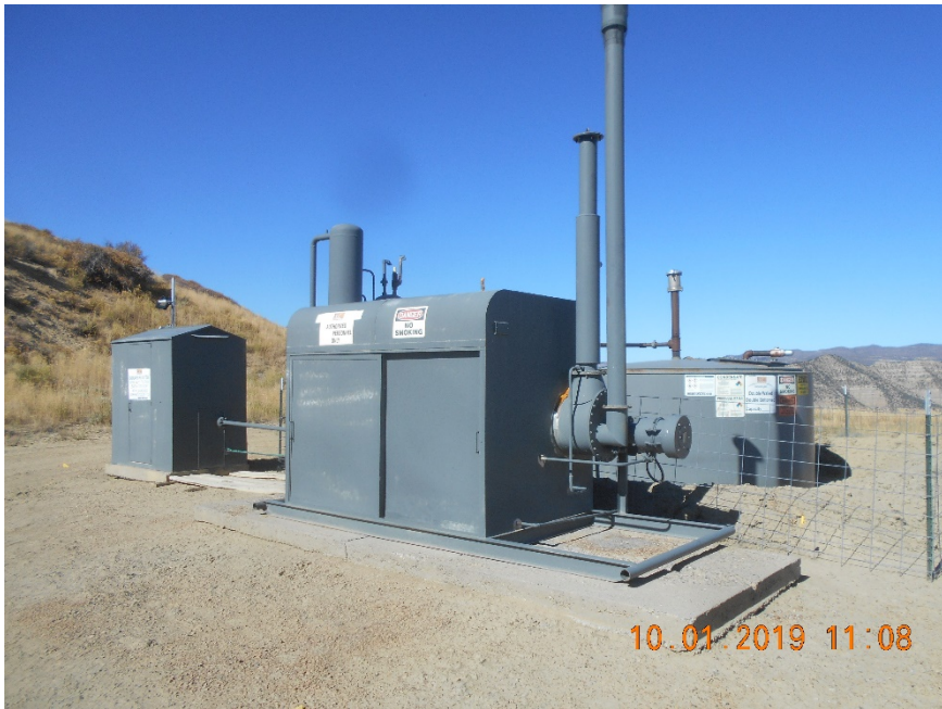
Separator and Meter Housing with sign
