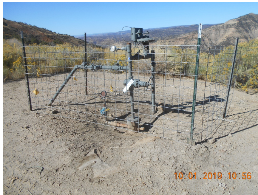
Wellhead with fencing.
