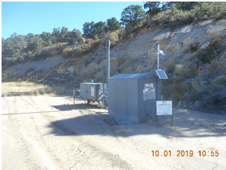
Separator and Meter Housing with sign
