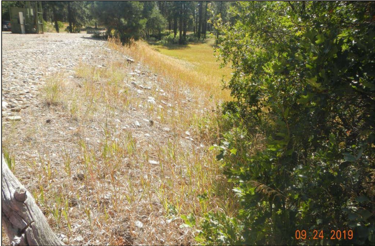
Photo 1. View of western fill slope from the northwestern edge facing southward. Revegetation is largely comprised of smooth brome and gambel oak trees.
