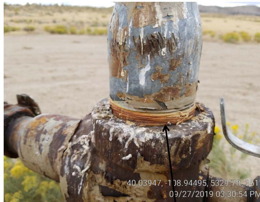
Photo 9. Well head gas leak.
