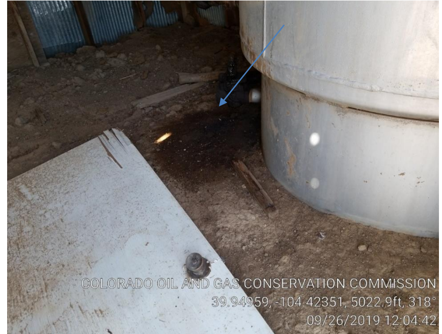
Pic 6 stained soil/mechanical issue
