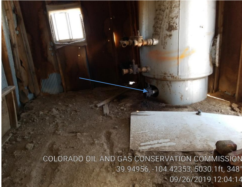
Pic 5 stained soil/mechanical issue
