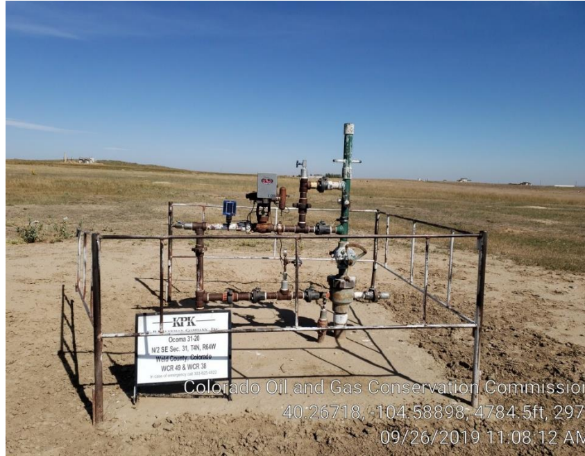
Photo #1 Wellhead & Sign
