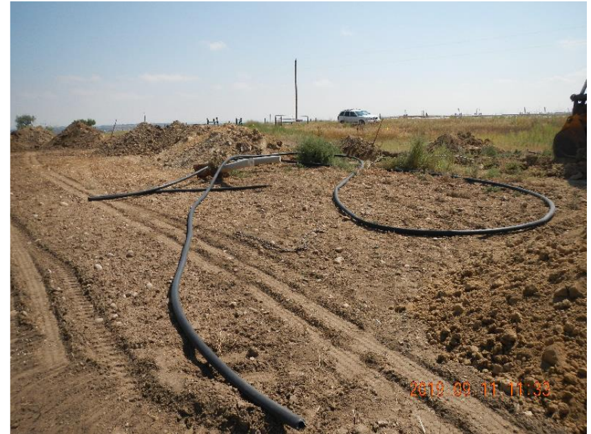
Photo 8: Removed black poly flow line prior to cut up and haul off.
