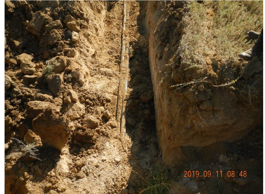
Photo 4: Excavation trench with flow lines in the bottom heading W towards old separator site.
