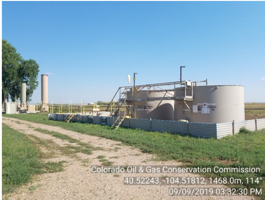
Photo #3 Dyer 2-21, 2-24, 2-25 Battery Shut-down | Inactive prior insp.
