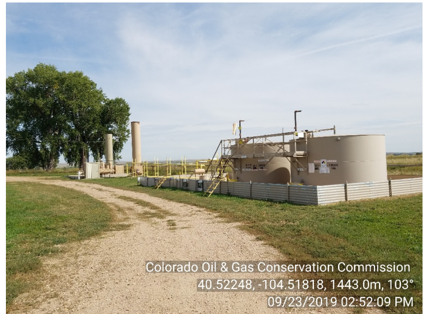
Photo #4 Dyer 2-21, 2-24, 2-25 Battery Shut-down | Inactive
