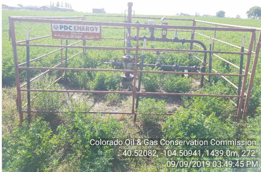
Photo #1 Cecil 41-2 (05-123-22707) Wellsite Shut-In | SI Weeds prior insp.
