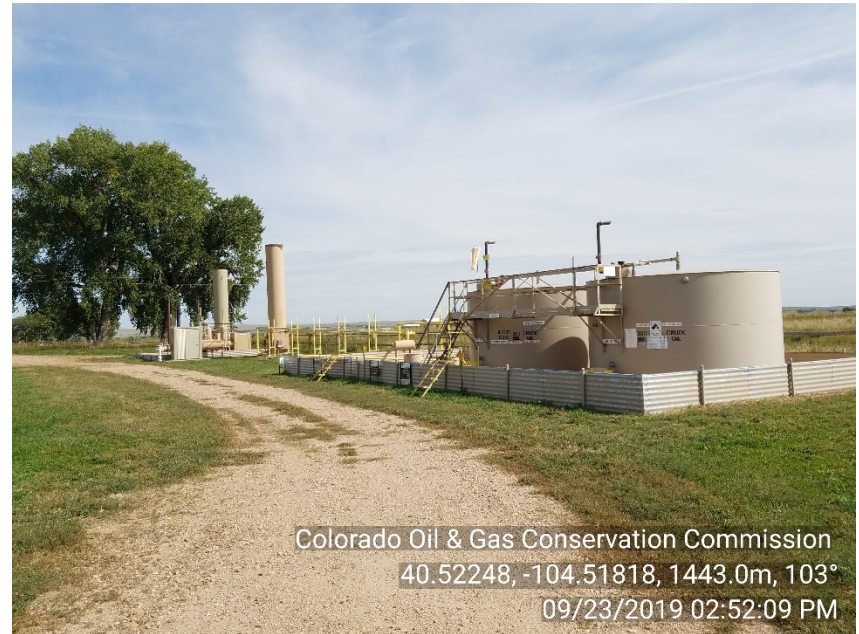
Photo #2 Dyer 2-21, 2-24, 2-25 Battery Shut-down | Inactive
