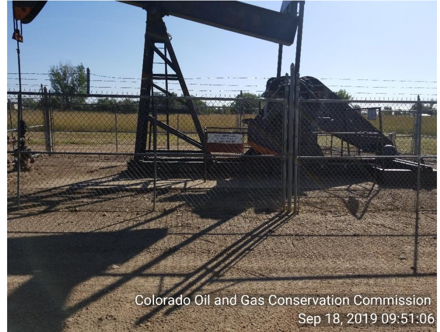
Photo 2 PU and well head. Installed sticker over old sign
