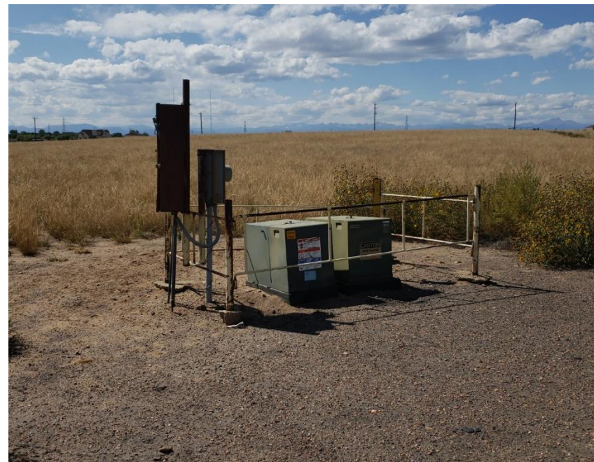
Photo #2 electric transformers, electric panel and meterbox.
