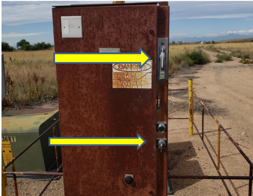
Photo #1 Electric panel appears to be shut off
