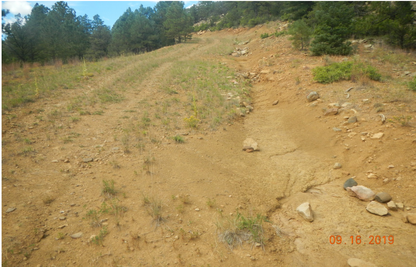
Photo 2. There is erosion issues along the access road as it ascends the hill.
