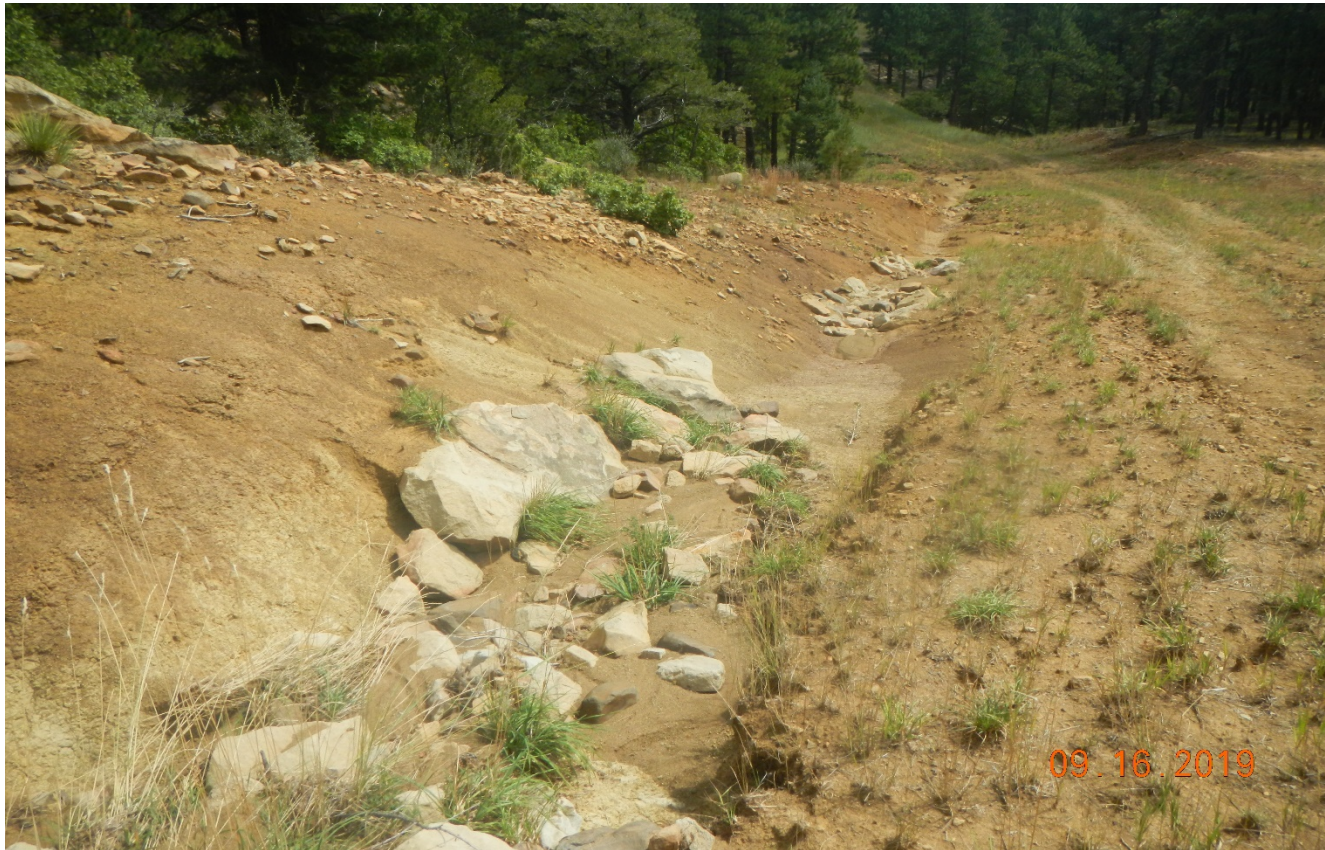
Photo 4. There are no BMP's to prevent erosion on the side of the road. It looks like check dams have been displaced.
