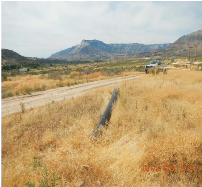
Photo from inspection Document Number: 689703459,
