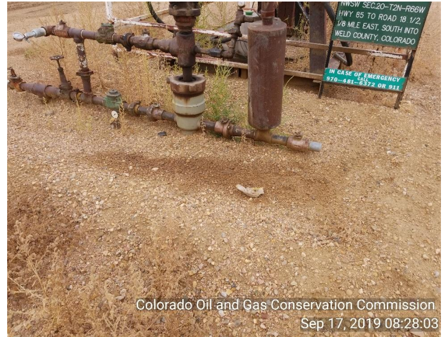
Photo 2 Weeds and stained soil around well head
