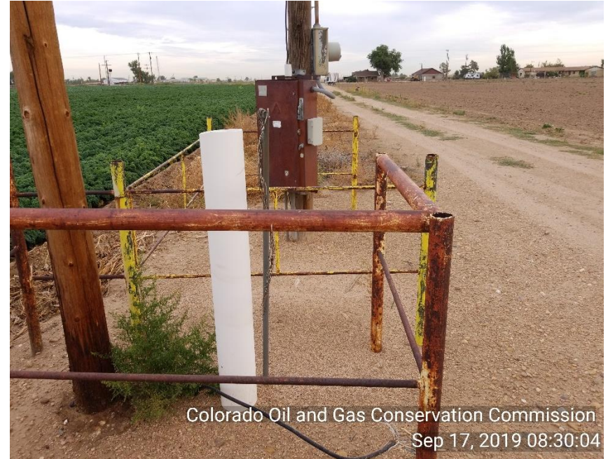
Photo 6 Electric panel for PU is in the off position. Unused equipment: electrical wiring sticking out of ground.
