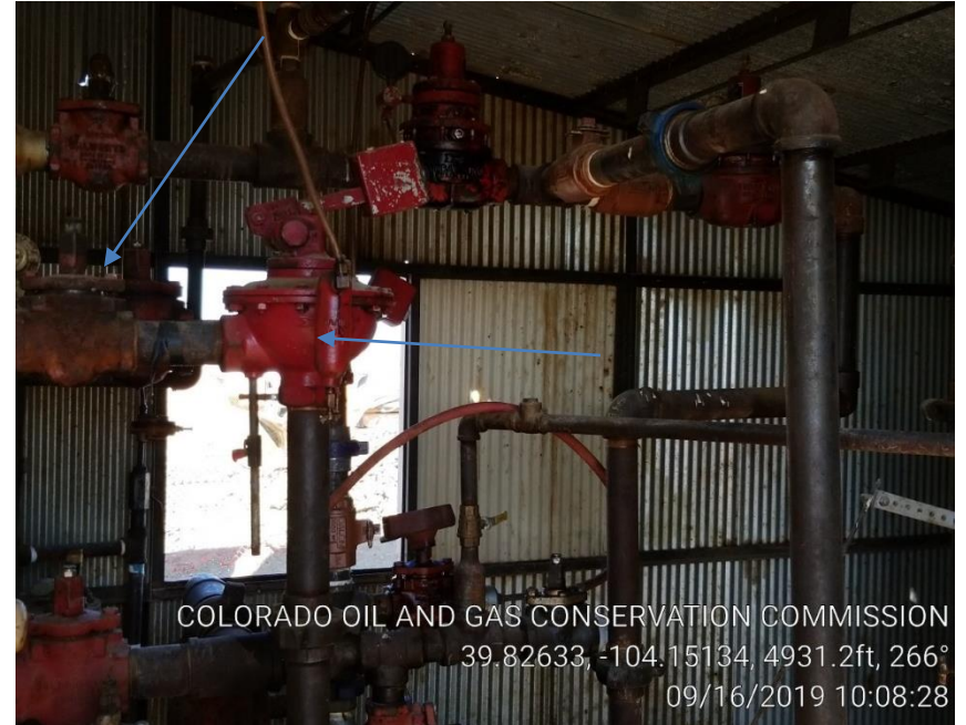
Pic 16 mechanical conditions in separator house
