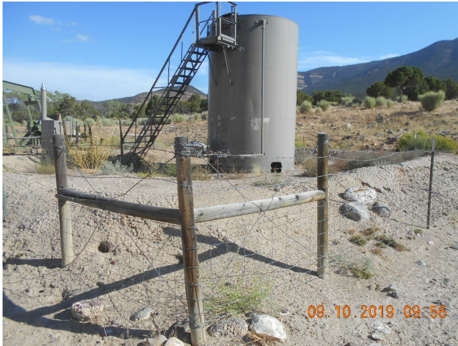
Tank battery with earth berms and fence. Looking N.
