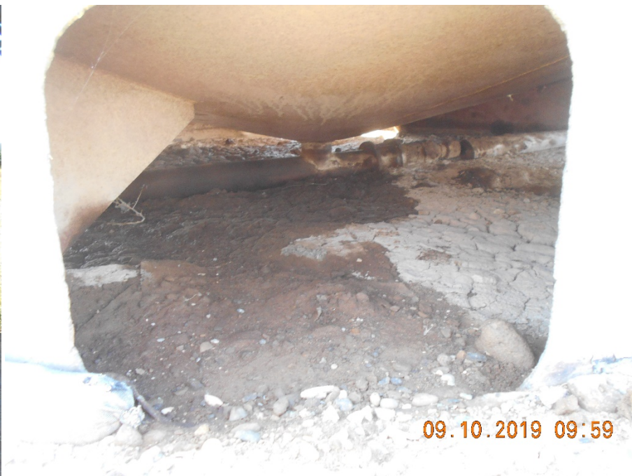
Leaking fitting at base of tank. Looking into inspection opening.
