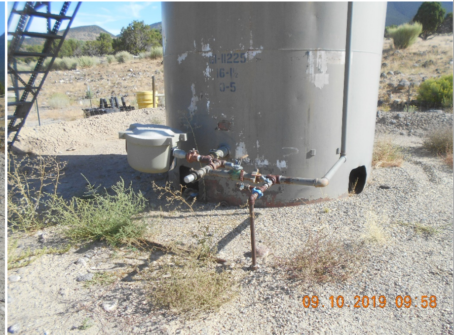
Weeds inside tank berms.
