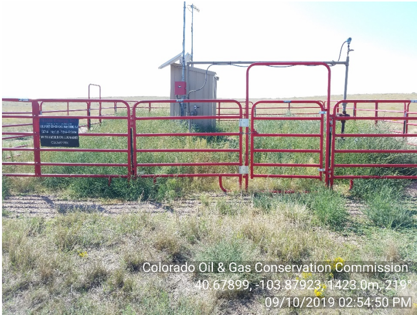
Photo #1 Lilli Unit 8-8 (05-123-13862) UIC - Injection Wellsite UIC Annual Inspection Not Injecting - Gas Shut-In | SI Weeds
