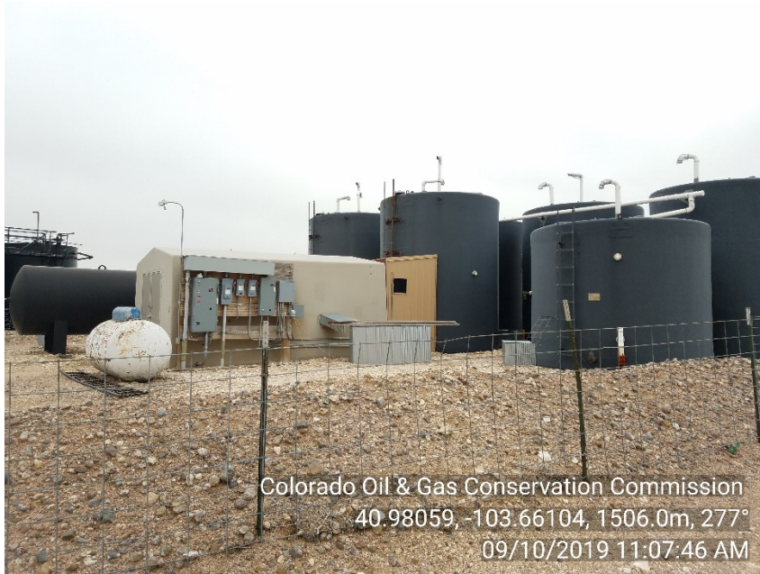
Photo #5 Moyer Unit Battery Free Water Knockout UIC Injection Facility
