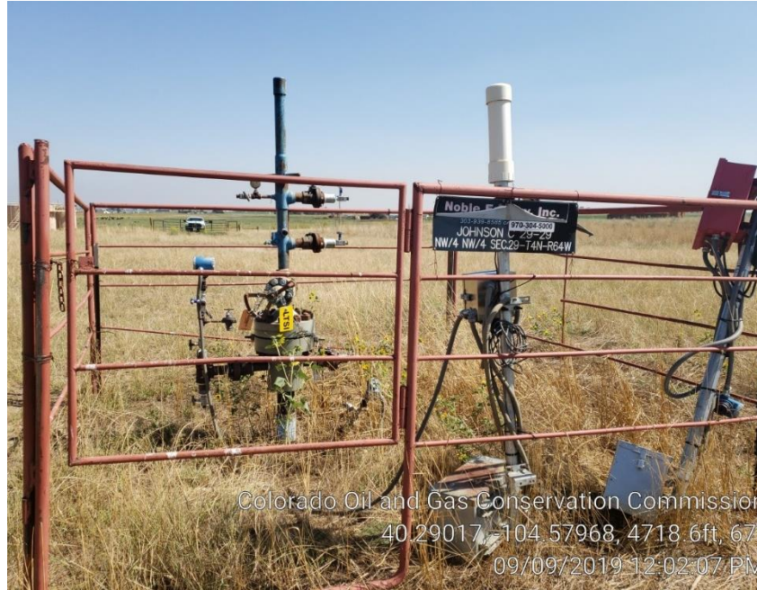
Photo #1 Well & Sign
